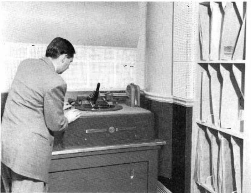
FIG. 3. Photos at left show two views into the combined recording room and studio A control room. Control equipment consists of an RCA Type 76-C Consolette and Type BCS-1A Studio Switching unit. Lower photo shows the Type 73-B Professional Recorder in use.
